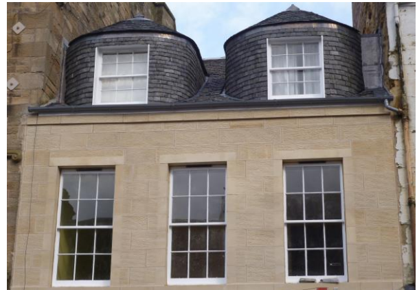
Completed Building Repair Grant Scheme project at 39/41 Bonnygate (masonry repairs, repairs to rainwater goods and roof repairs):
